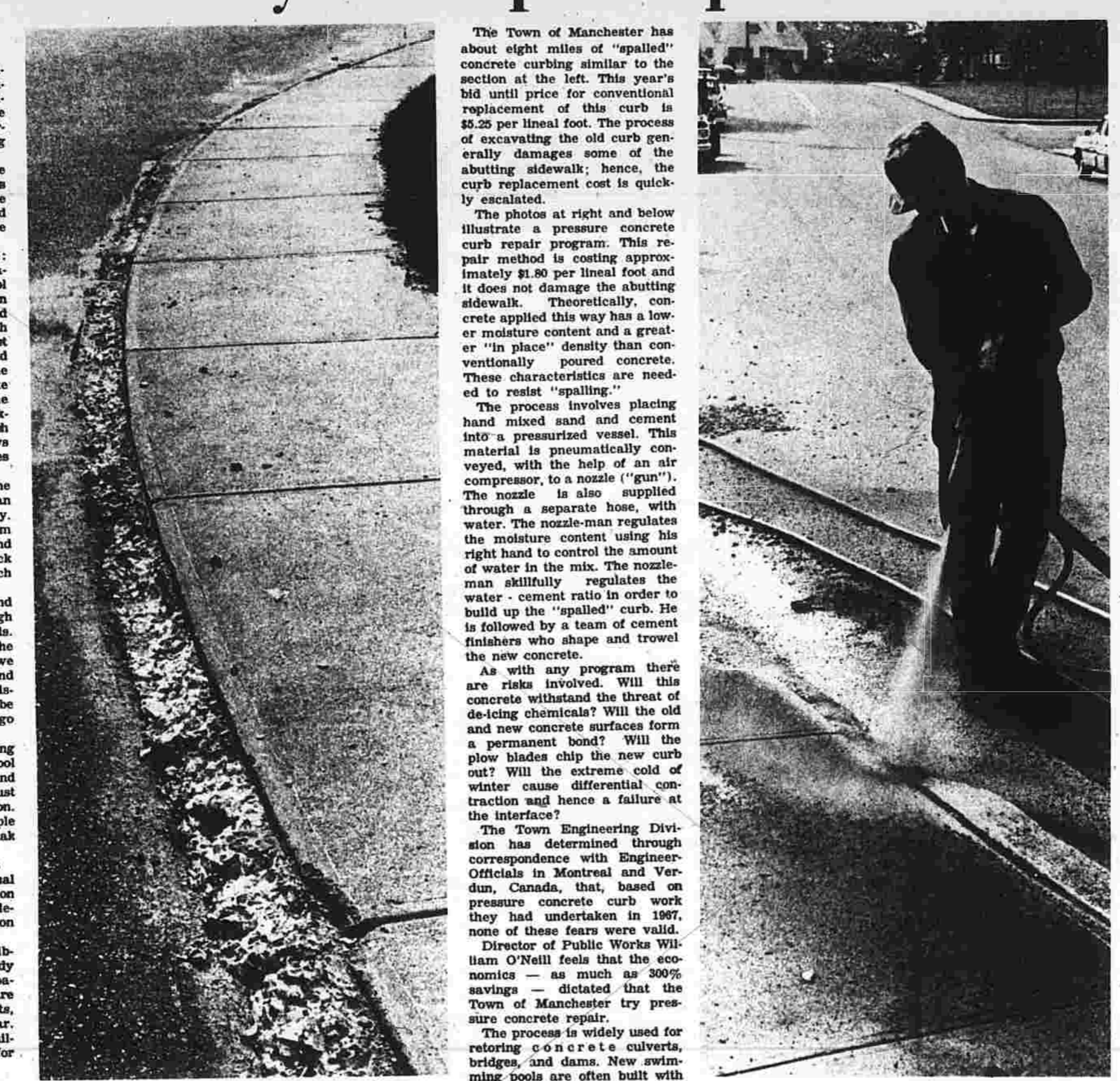
The Town of Manchester has about eight miles of 'spalled' concrete curbing similar to the section at the left. This year's bid until price for conventional replacement of this curb is $2.25 per linear foot.
